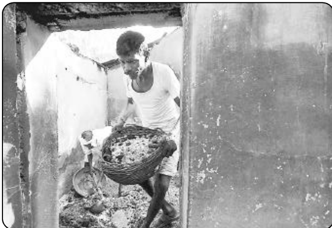
Charred debris being cleared from the house where six Muslims were burnt alive on Oct. 10, 2008 in Vatoli village near Bhainsa in Adilabad district of Andhra Pradesh
